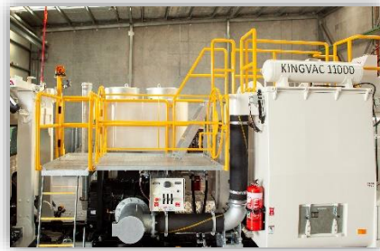
Image 36 - Platform on top of the blower
