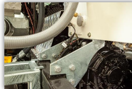
Image 25 - Low water level cut-out switch
