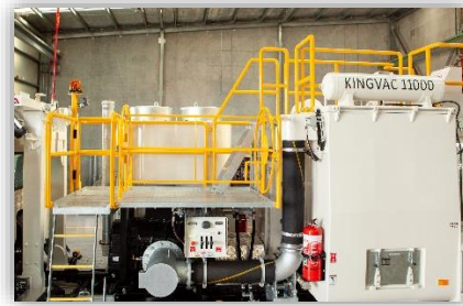
Image 36 - Platform on top of the blower
